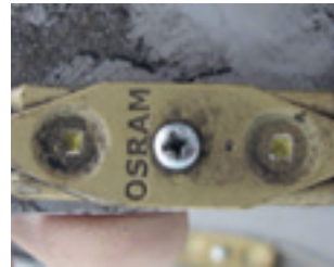
Dirt on top of the LED surfaces
